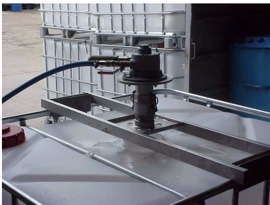
Air driven mixer motor with bridge assembly
